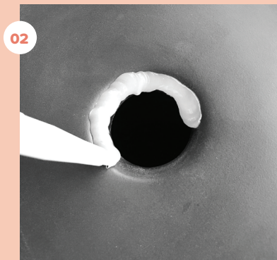
02 Be generous with application. It is critical that silicone overflows when waste is placed down
